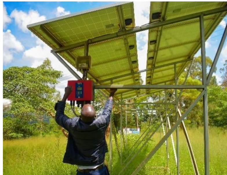
The solar system for pumping
